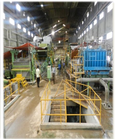
CLIENT: BGDCL ASSOCIATE: MACDOW GAS PROCESSING FACILITY MECHANICAL
