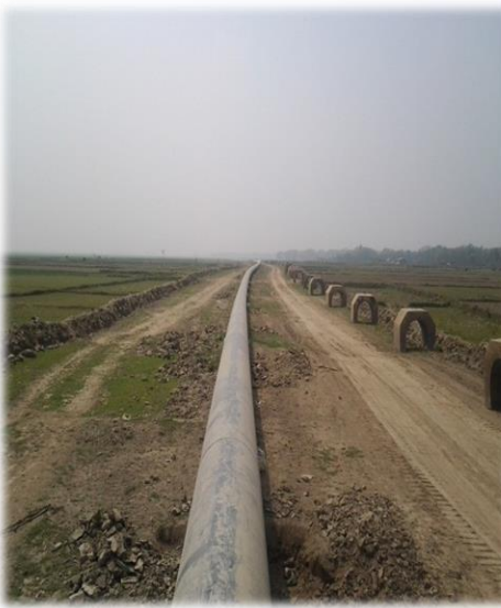
CLIENT: GAS TRANSMISSION COMPANY LIMITED (GTCL) CONSTRUCTION OF 36" OD HIGH PRESSURE GAS TRANSMISSION PIPELINE
