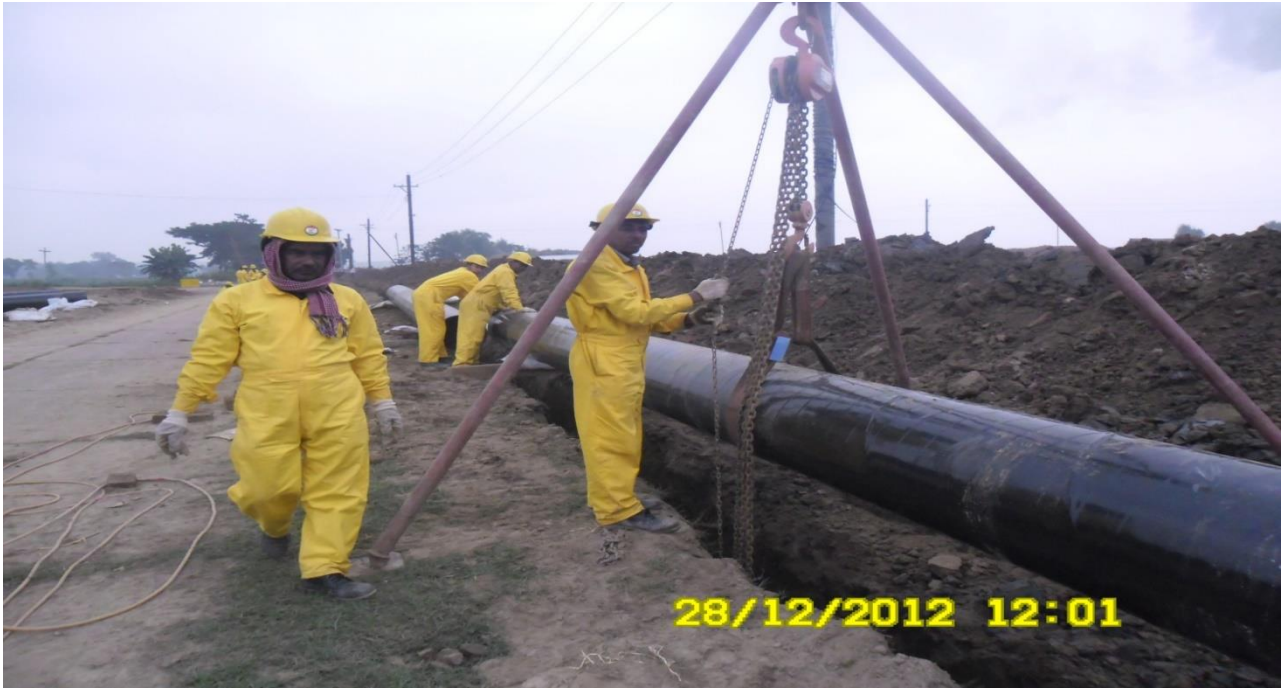
Construction of 20"OD 4 KM River Water Intake Pipeline at SFP, Fenchugonj, Under COMPLANT, China
