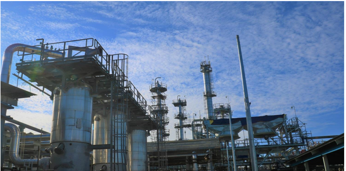
Installed Equipment in CRU Project, Hobiganj.
