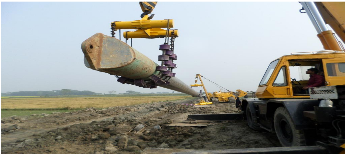
20" OD X 1250M Pipeline Hanging to Over bend for Pulling beneath Kornophully River for crossing by HDD under Mershing Construction, Malaysia.
