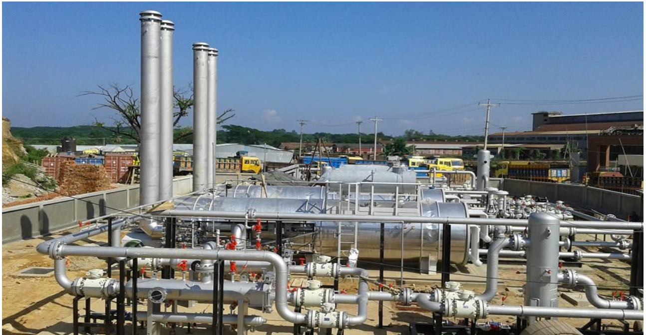
Turnkey Construction of 70MMSCFD RMS Station at Shajalal Fertilizer under Valvitalia, Italy.
