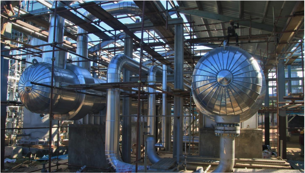
Installed Equipment & Piping for CRU Project, Habiganj
