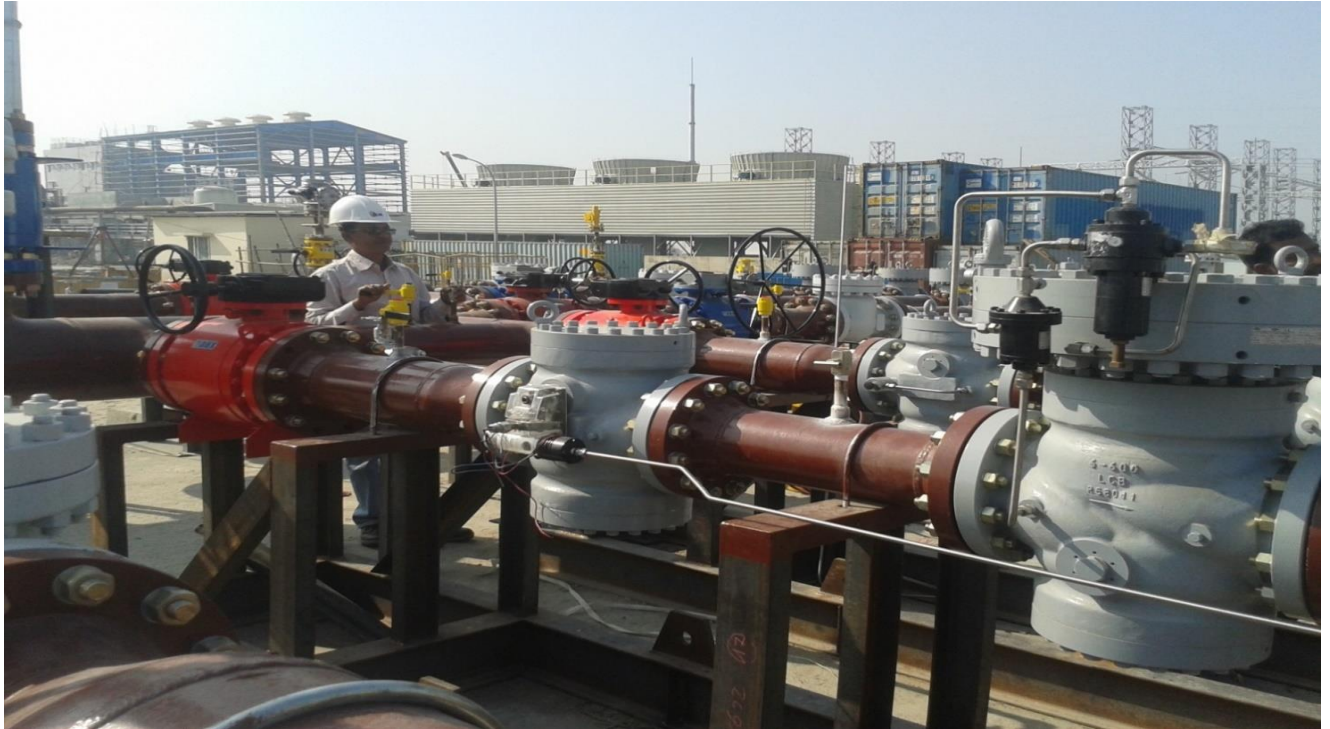
Fabrication, Installation, Testing & Commissioning of 40MMSCFD CMS at 225MW CCPP, Bhola under PDB
