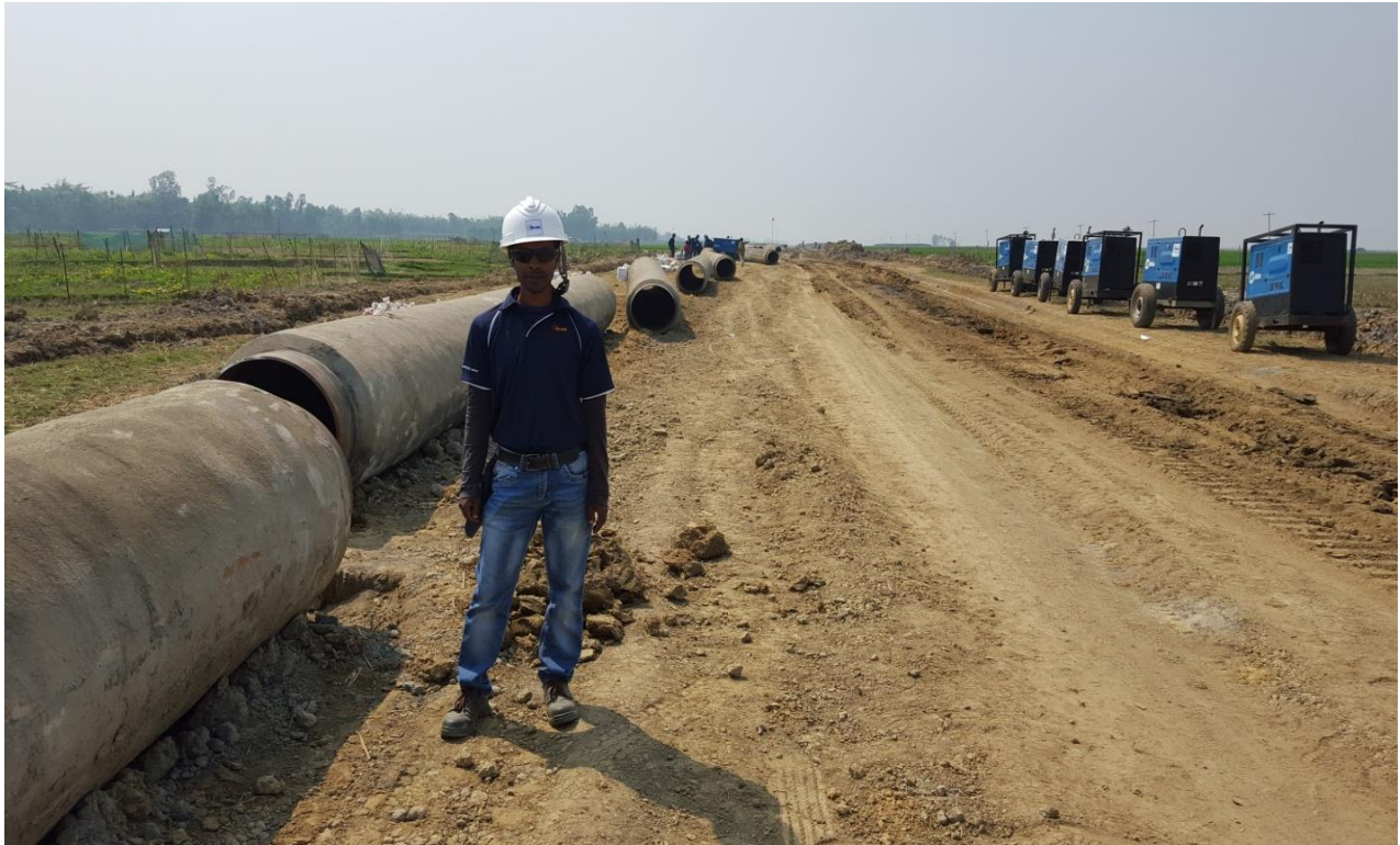
Stringing of RCC Coated Line pipe along ROW of Anwara-Maheshkhali 30inch Diameter LNG Transmission Line
