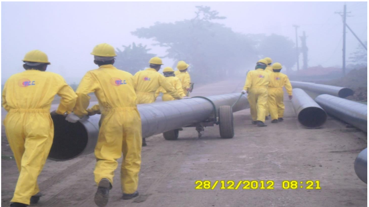
Construction of 20"OD 4 KM River Water Intake Pipeline at SFP, Fenchugonj, Under COMPLANT, China
