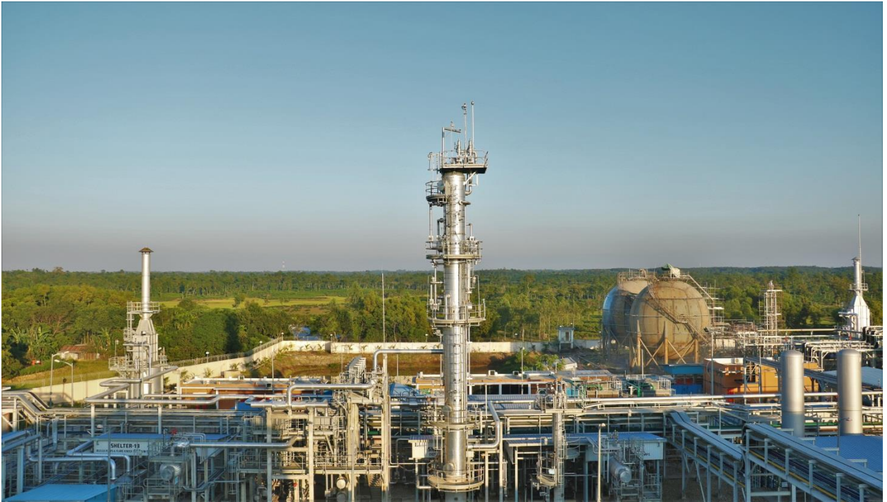
Catalytic Reforming Unit (CRU) Plant In Habiganj.
