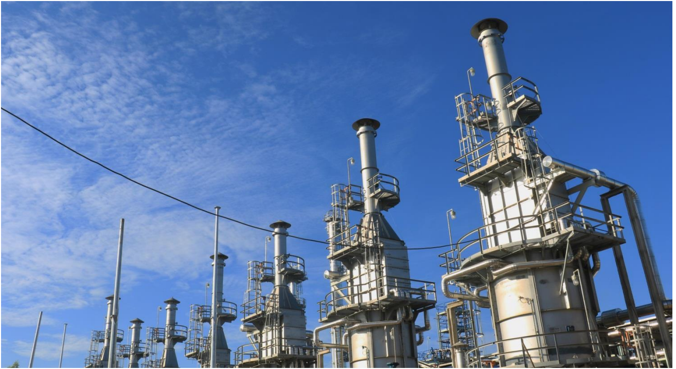
Installed Heater for Catalytic Reforming Unit (CRU) in Habiganj.
